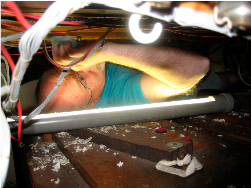
TOSA NSW Vice President Neil Palmer works on the Orchestral Oboe Chest in situ at Marrickville replacing secondary motors
