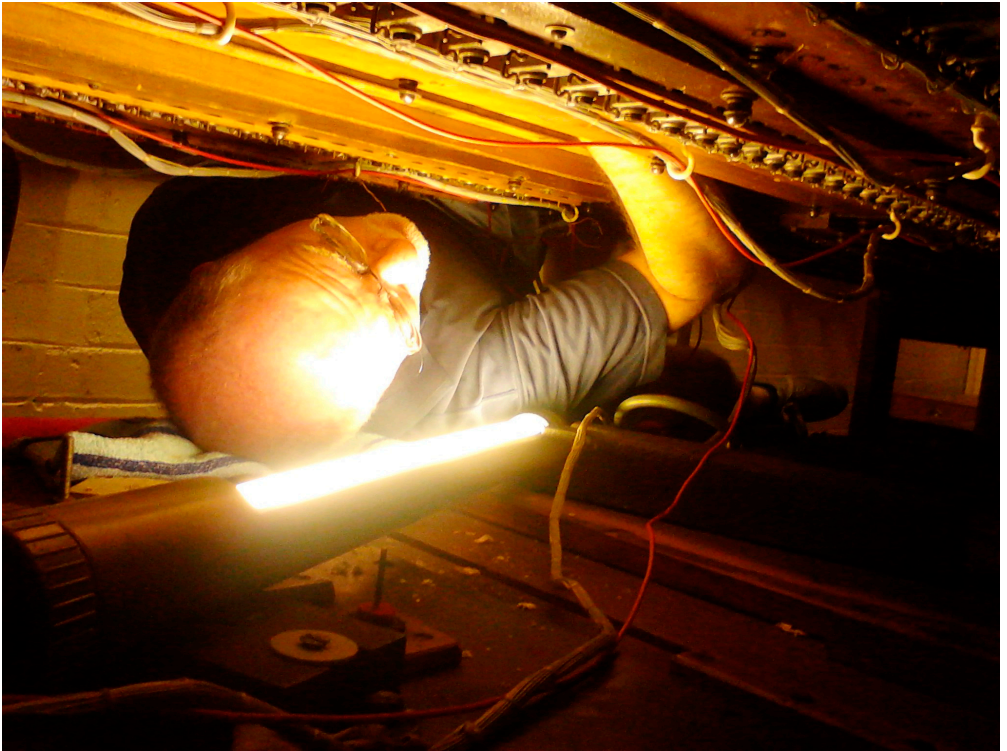
Neil Palmer under the Oboe Chest at Marrickville Town Hall cleaning off the old gasket before replacing a secondary motor
