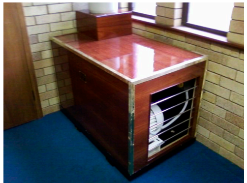
THE MUFFLER BOX FOR THE CHRISTIE BLOWER
