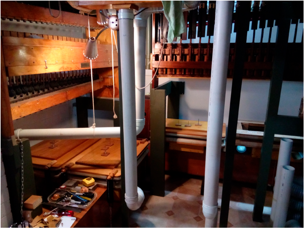
Fitting of the Regulators in the Accompaniment Chamber maximising the use of the minimum space available. Several chests attached to wind to test the ranks and identify any ciphers
