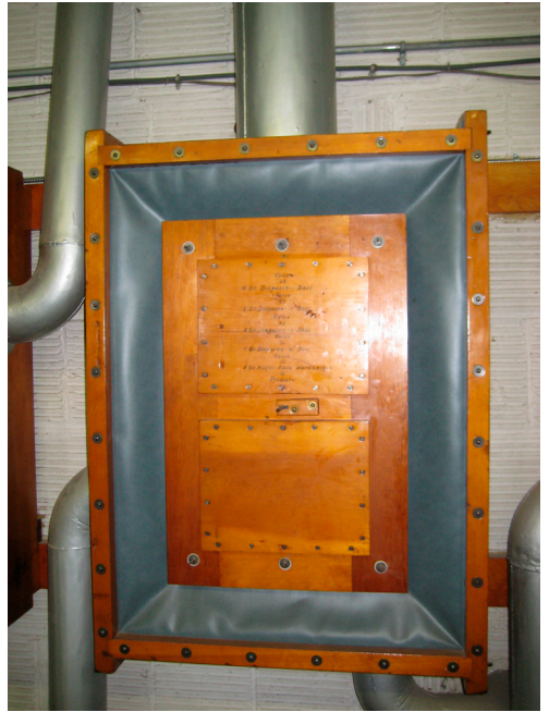
One of the regulators outside the chamber
